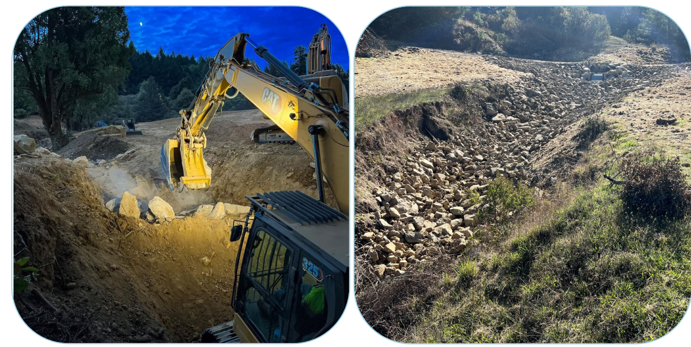
A previously deep gully now has grade control, is now part of the armored spillway and functions as a cooling/infiltration gallery.
