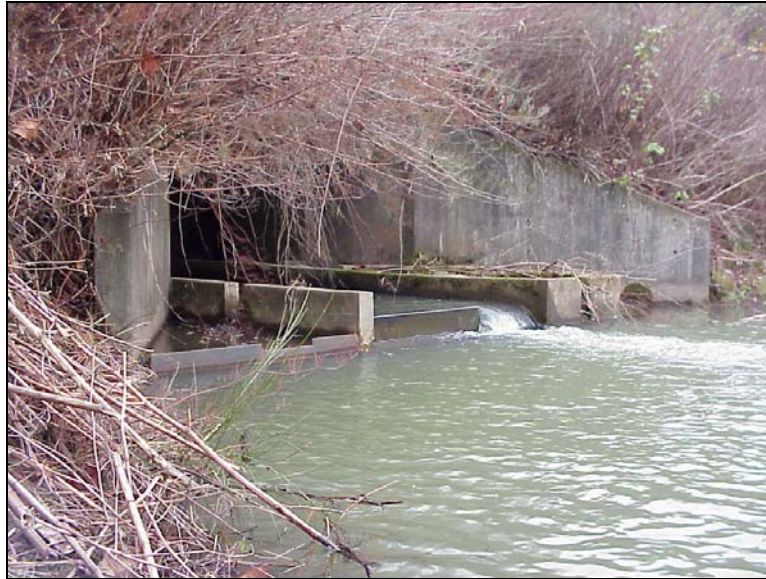
Figure 7-8. Enhancements at box culvert outlets might include training walls and notched weir sills to maintain flow depth in the main channel section, along with secondary entrances to promote better conditions for juveniles during higher flow conditions. (Photo courtesy of ODOT)
