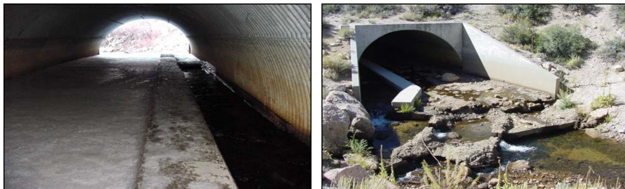
Figure 7-2. Longitudinal channel weir and grade control rock weirs at the Crooked Creek retrofit project.
