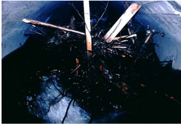
a) debris caught on baffle
