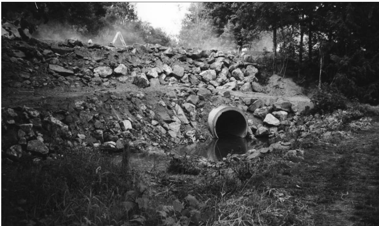
Figure 6-1. Outlet view of a culvert replacement project developed through the hydraulic design option.
