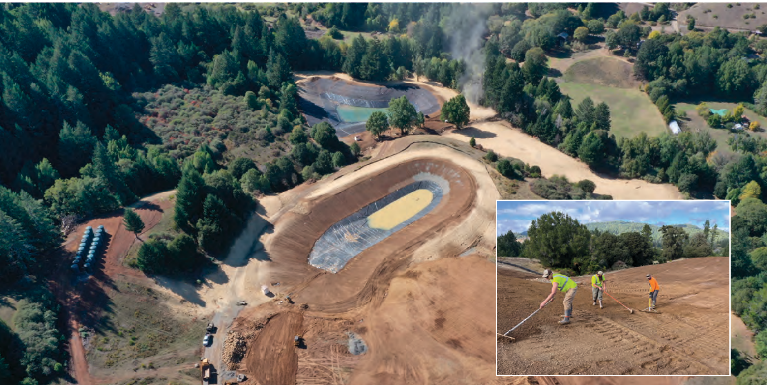
Drone photo of the recently completed lined ponds and the meadow area that was reseeded with native grasses.
