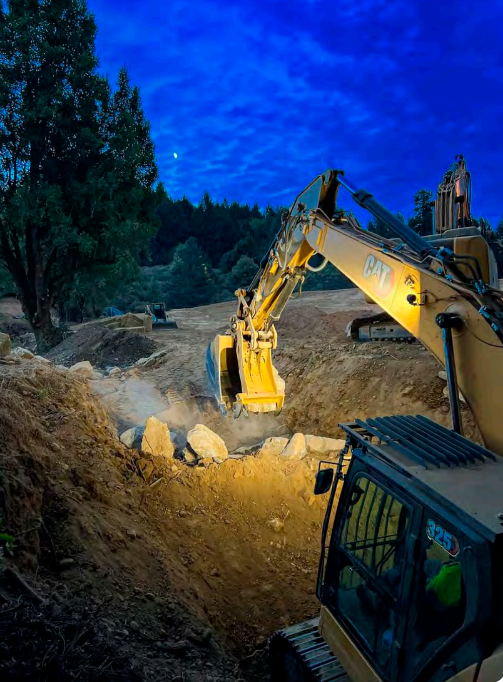
Creating grade control structures on the cooling gallery. PHOTO BY JOAQUIN COURTEMANCHE
