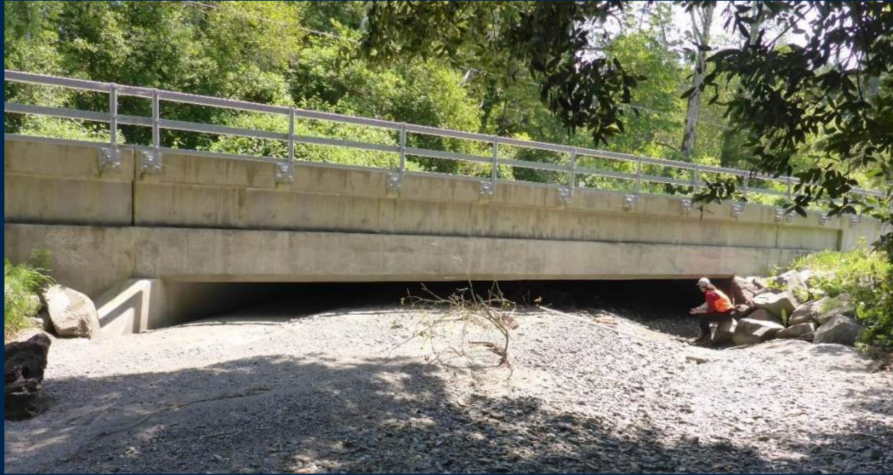
Sultan Creek Bridge Influenced by River Backwatering
