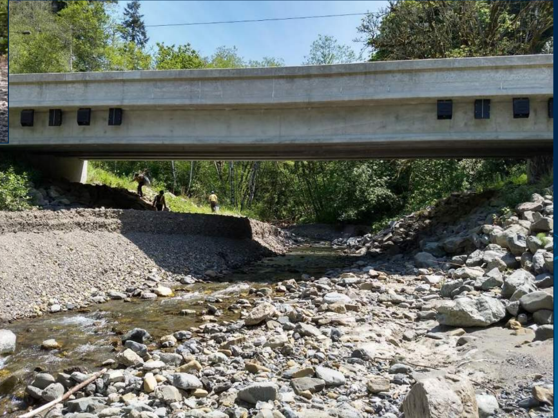
Little Mill Creek Bridge Depositional Bar from River Backwatering
