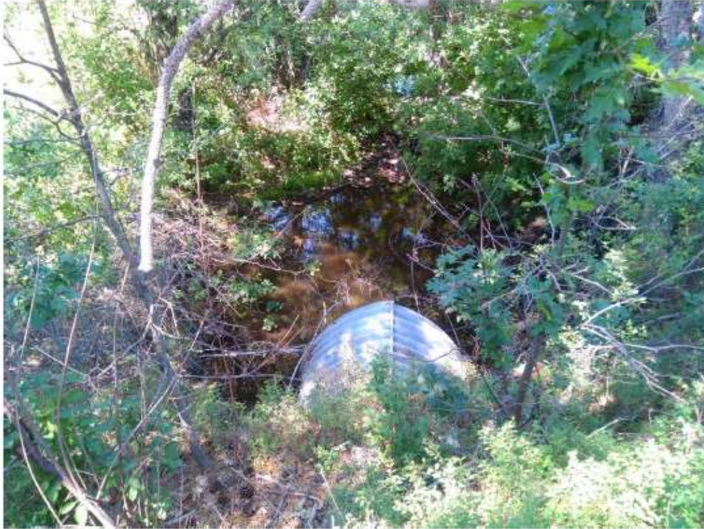
Figure 47. Looking downstream from the road at the Ager Beswick culvert on Deer Creek on 06/25/2021.
