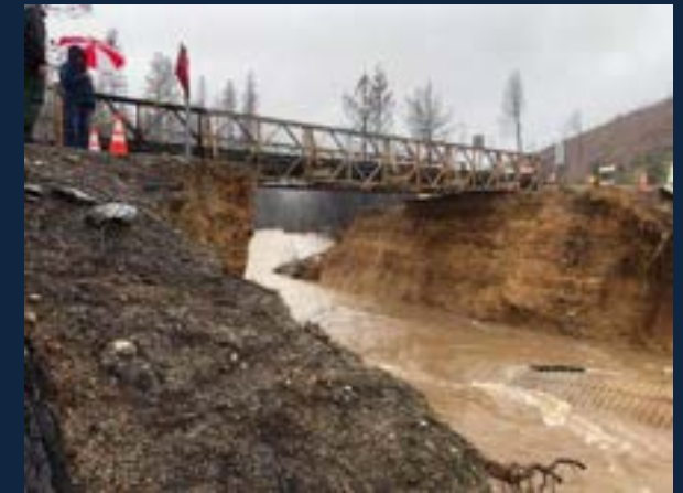
Whiskey Creek bridge loss, 2018 Carr Fire
