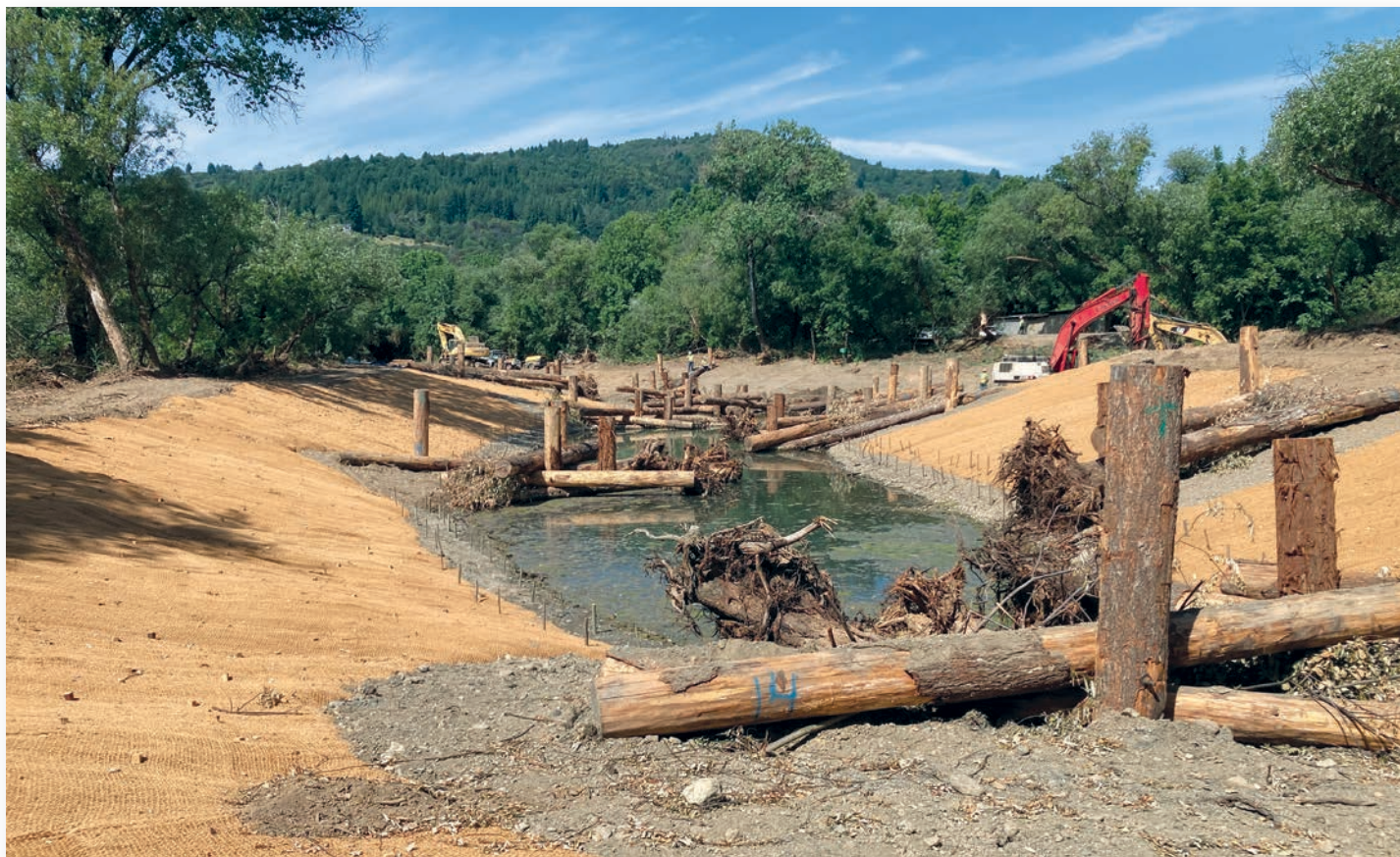
A Dry Creek habitat enhancement under construction on private property. This project was built by McCullough Construction. Implementation of the project was managed by the USACE. The photo of this newly constructed project was taken during the 2023 construction season. Credit: Justin Smith
