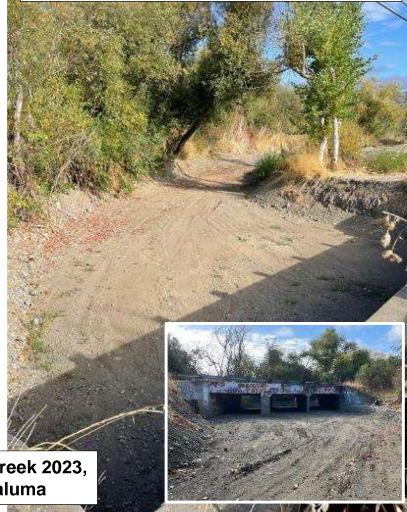
Sediment removed from culverted road crossing
