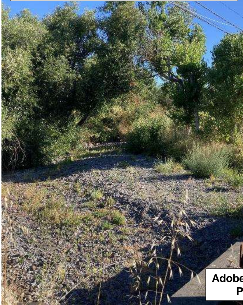
Sediment obstructing culverted road crossing
