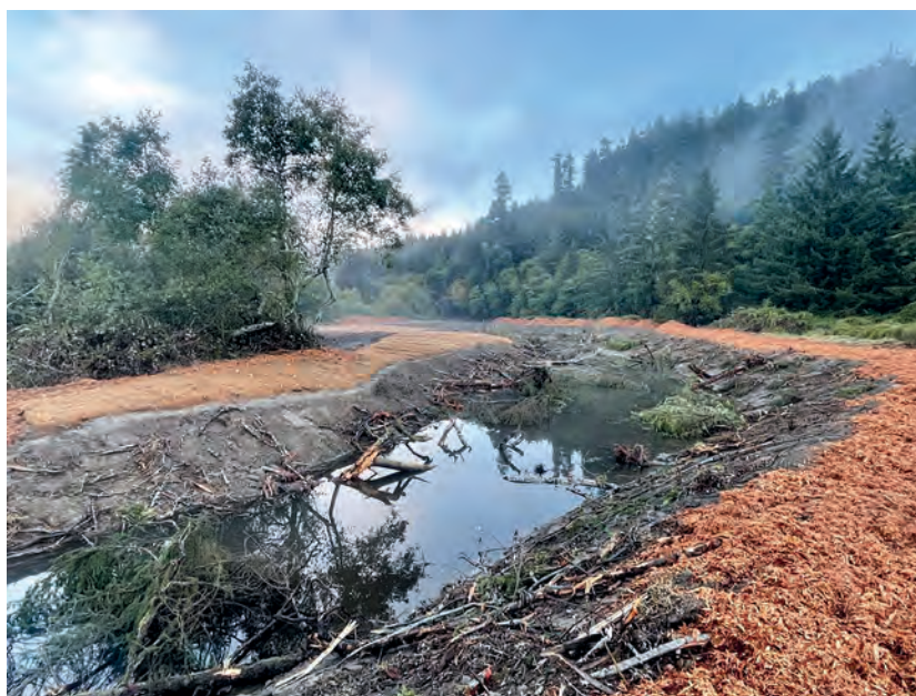
The Lower Prairie Creek Early Implementation Pond shortly after construction Photo credit: Bob Pagliuco
