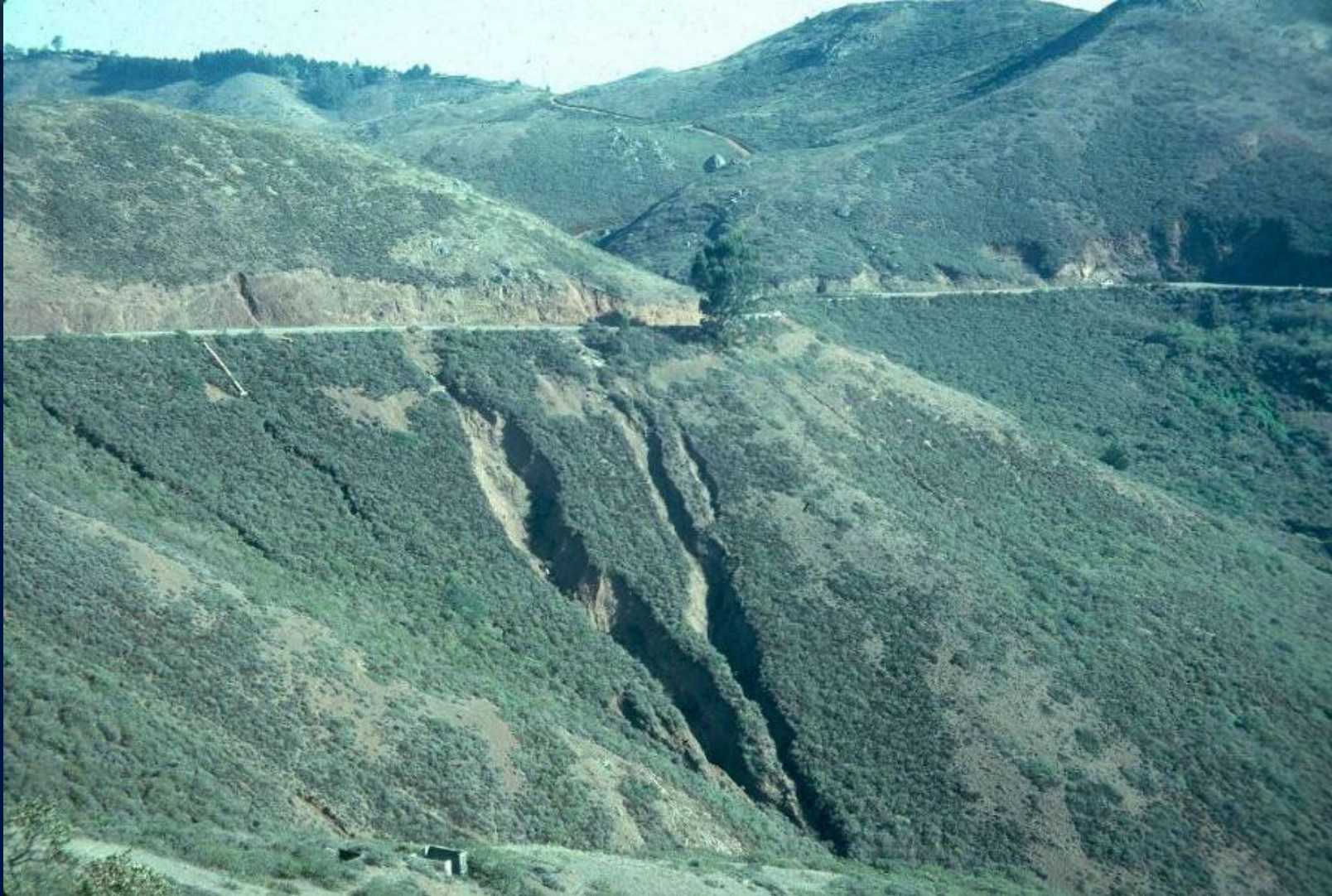
Gullies from road surface runoff
