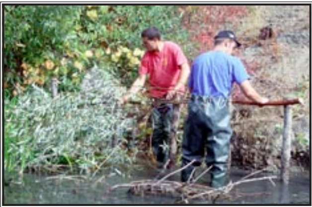
Installing a live woven willow wall to stabilize and revegetate an eroding bare stream bank.
